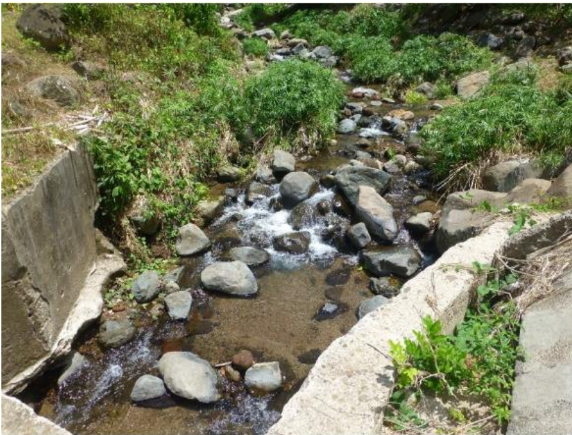
Figure 9.5: Mt Reuil Stream looking upstream from culvert adjacent to the Glenelg bottling plant.
