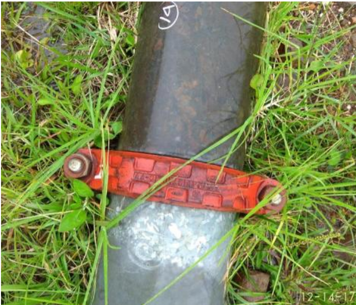
Figure 2.10: Example of temporary carbon steel water pipeline with connection clamp in geothermal drilling
