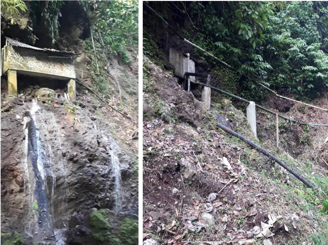
Figure 9.23: Glenelg upper (left) and lower (right) spring collection tanks and gravity feed pipework
